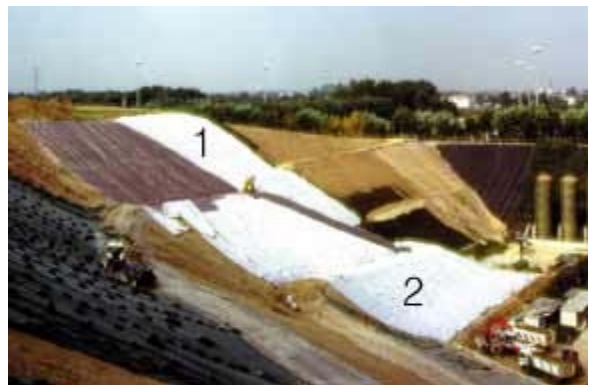
Cerro Maggiore (Italy) - Landfill capping 1: TENAX geocomposites for rainfall drainage 2: TENAX geocomposites for biogas drainage
