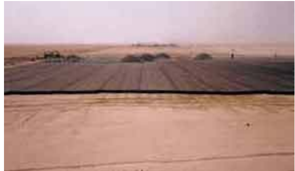
Geogrid layers during rock fill operation. The overall project required 700,000 m 2 of TENAX LBO 303 SAMP
