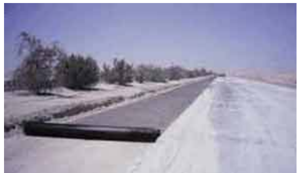
TENAX geogrids rolls are 100 m long and are ideal for highway projects with all soil conditions
